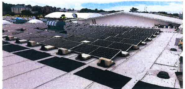
We designed the roof replacement and PV system on E.O. Smith High School in nearby Mansfield.
