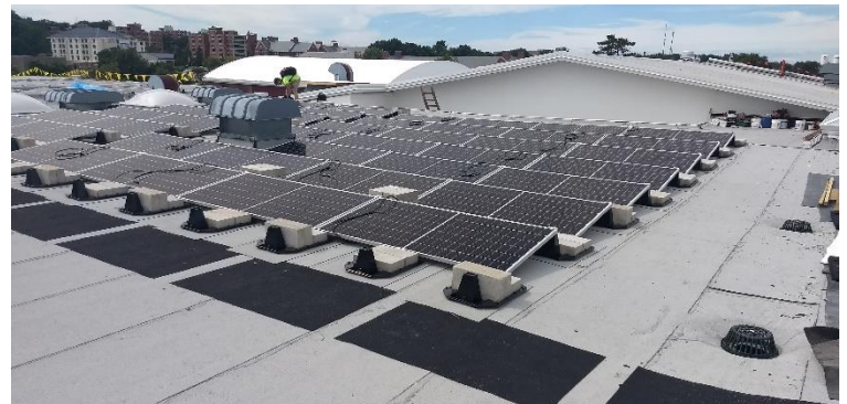
We designed the roof replacement and PV system on E.O. Smith High School in nearby Mansfield.
